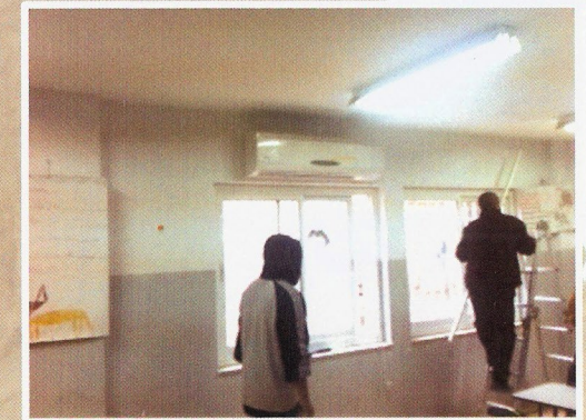
A/C unit in a classroom
